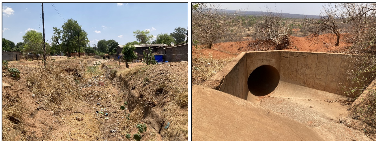
Figure 4.4: Victoria Falls City storm drains Unmaintained storm drain (left) and main outlet to the Zambezi River (right)
